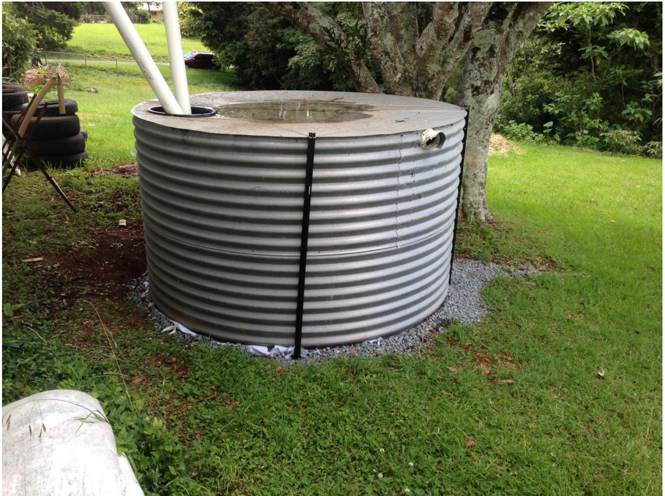
The Community Garden Group rainwater tank
